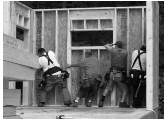
A new Olympic event? Four big guys setting a wall panel into place at Wild Rose Meadow.
