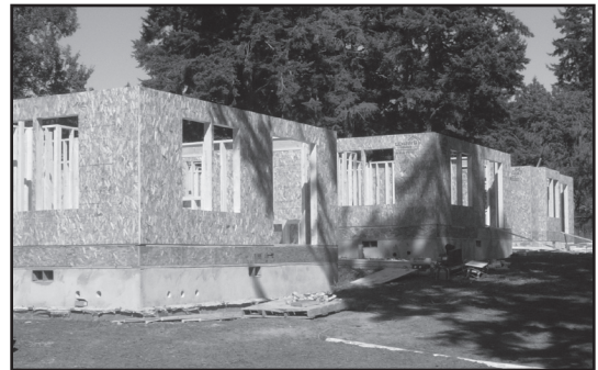
Panels arrived August 11; by midday August 13 five houses looked like these three. The Louws Truss crew takes about 1-1/2 hours to install panels for the exterior and put up inside walls in these one-bedroom homes.
