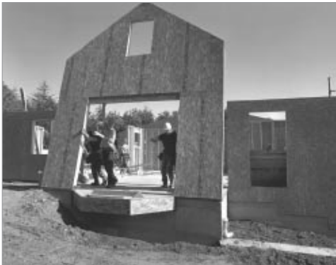
The south wall of the Farmhouse building is raised into place. The Farmhouse will contain a conference room, restrooms for the office spaces, and four small rental offices
